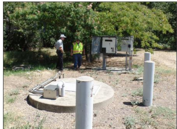
Photo 4: Quail Lane Lift Station
