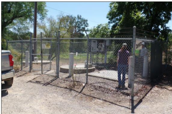
Photo 3: Black Lane Lift Station
