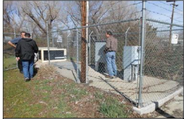
Photo 5: Crowley Creek Lift Station
